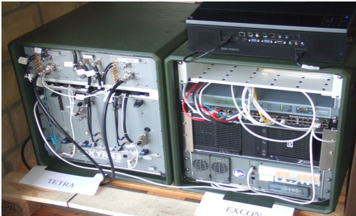
Figure 6-11: TETRA Radio Base Station and EXCON Workstation.
